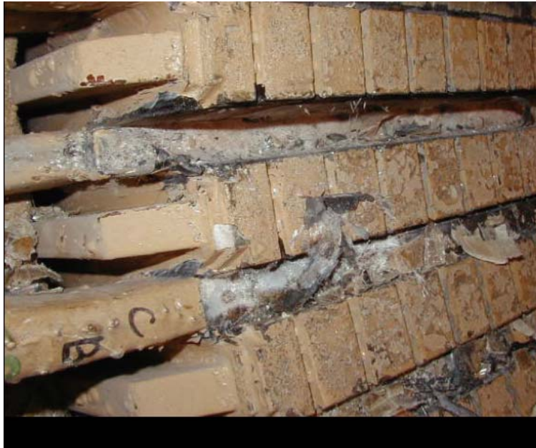
Figure 2. Stator winding failure on a 12,000HP, 13.8kV AC industrial motor.
